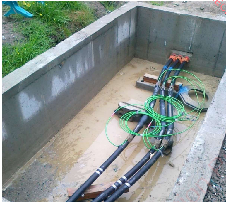
Plate 3.3 - A Typical Joint Bay
